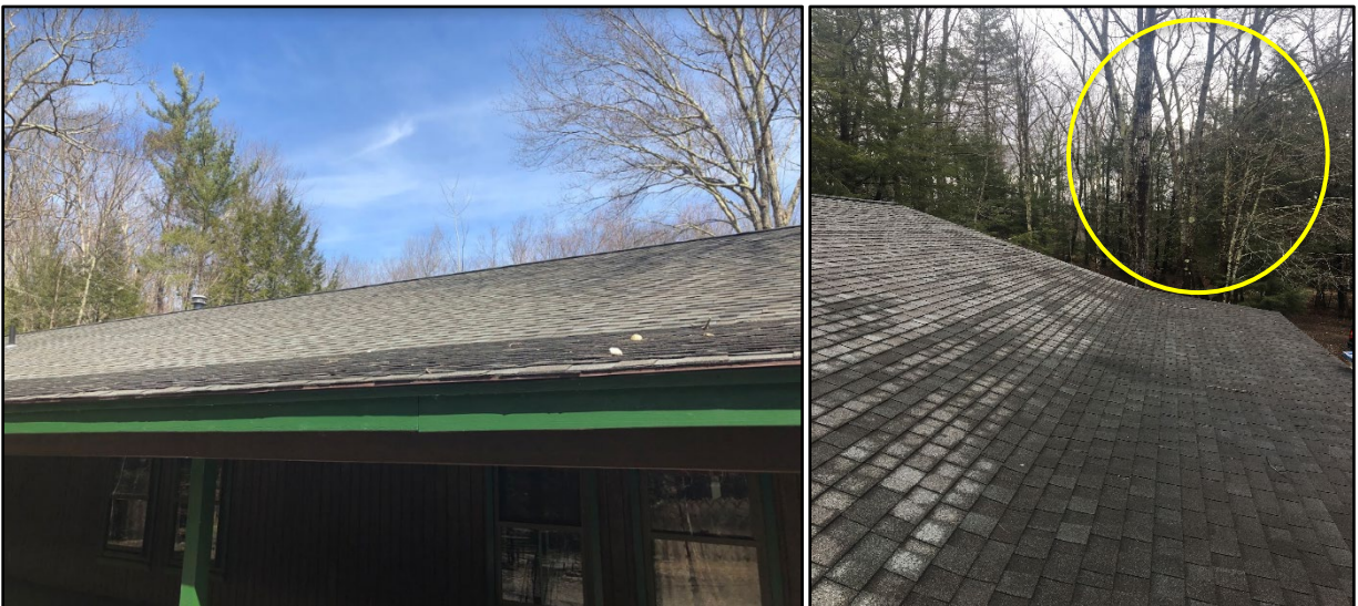
Figure 27: (a) Venture Lodge Roof and (b) Venture Lodge Roof with Tree Obstruction (Yellow)
