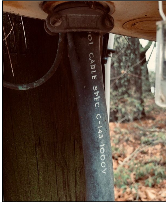
Figure 22: Pine Point Meter Power Cable
