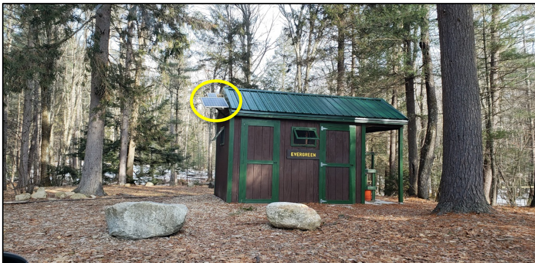
Figure 2: Camp Latrine with Solar Installment (Yellow)
