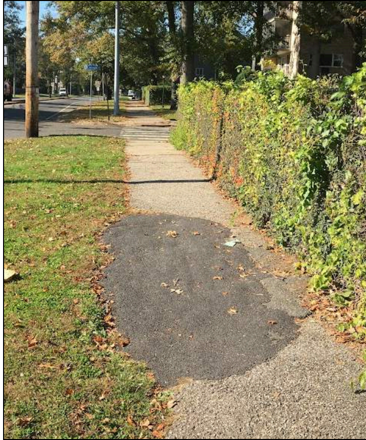
Figure 16. Unlevel Sidewalk Patching Conditions.
