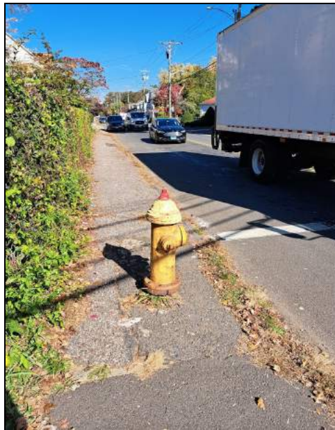
Figure 17. Fire Hydrant Obstructing Sidewalk on Briarwood St.
