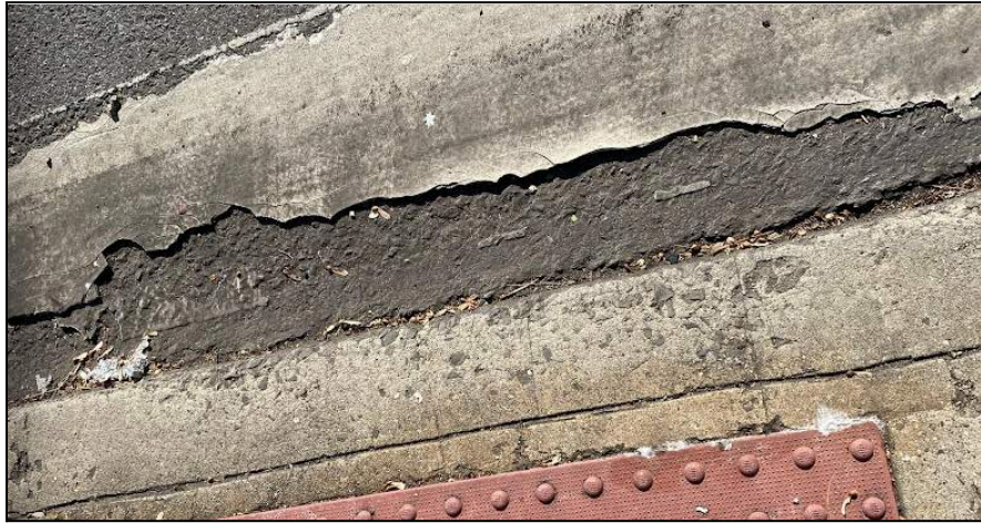
Figure 12. Deteriorating Crosswalk Paint.
