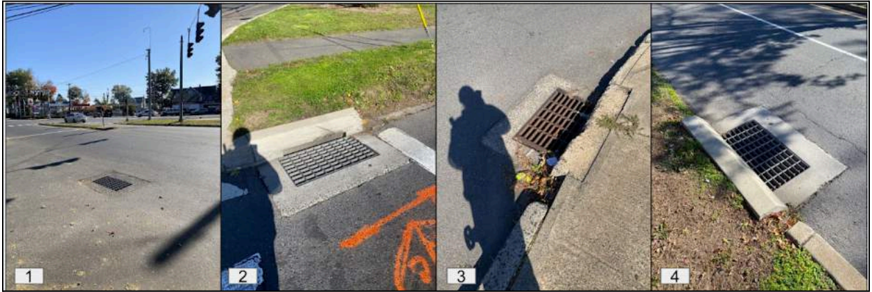
Figure 21. Conditions of the four catch basins in the vicinity of the intersection as labeled in Figure 20.
