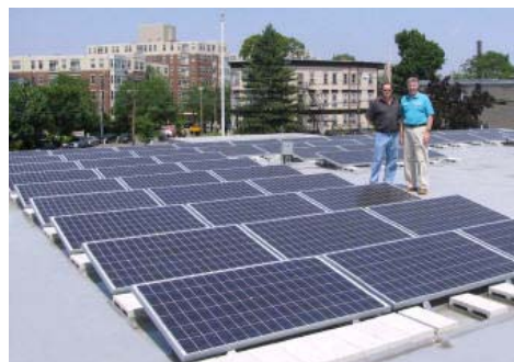
Figure 10: Flat Roof Array (Solar Flair, 2009)
