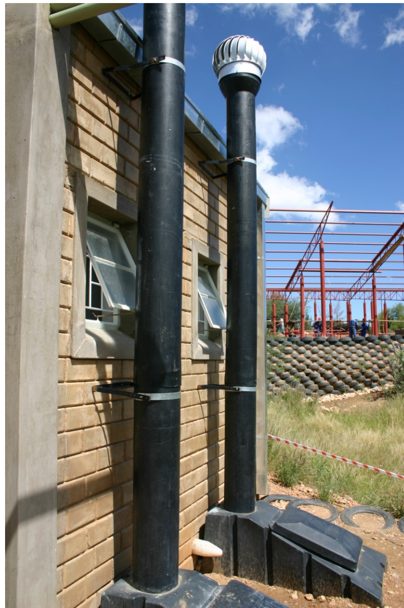
Figure 56: Outdoor waste storage utilized in the Enviro Loo design outside the Windhoek Habitat Research and Development Centre (March 17, 2004)
