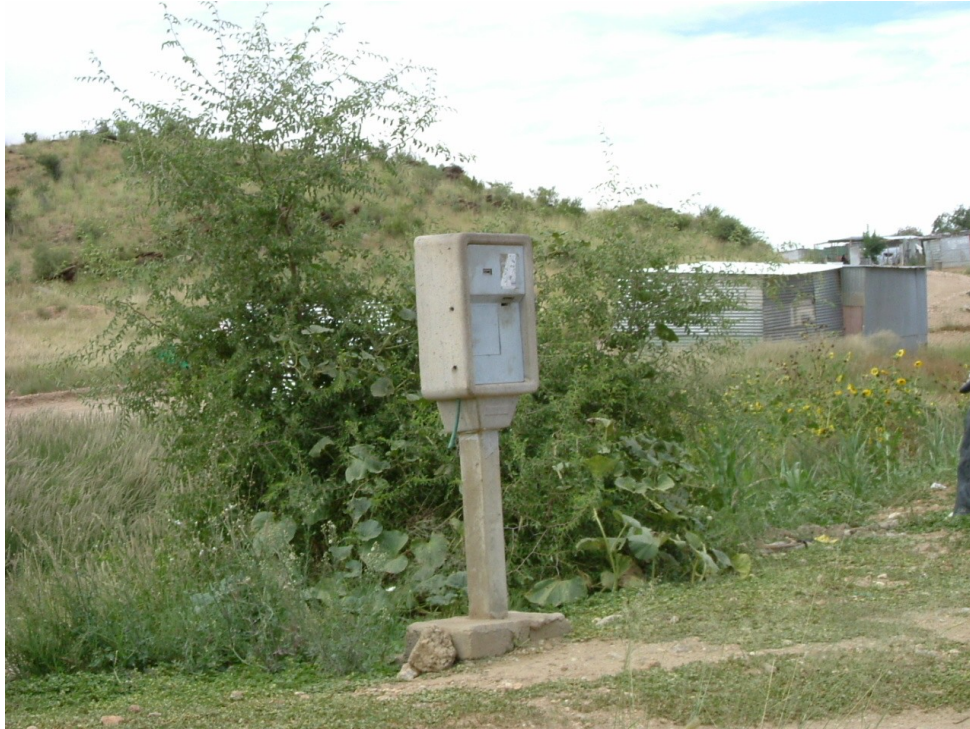
Figure 4: Prepayment water meter in Havana Northwest Settlements, Windhoek (16 March 2004)
