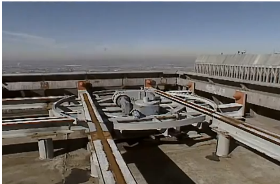
Figure 30: Window Washing Device (WTC: OCC, 2012)
