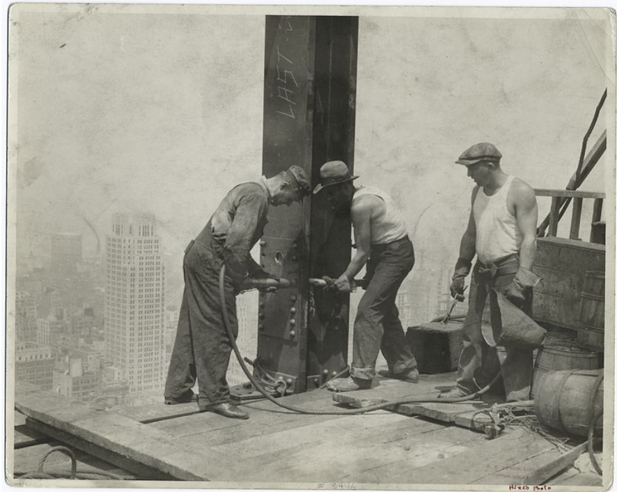
the office building. It can Figure 11: Construction Workers Connecting Columns (Vintage Photos, 2012)
