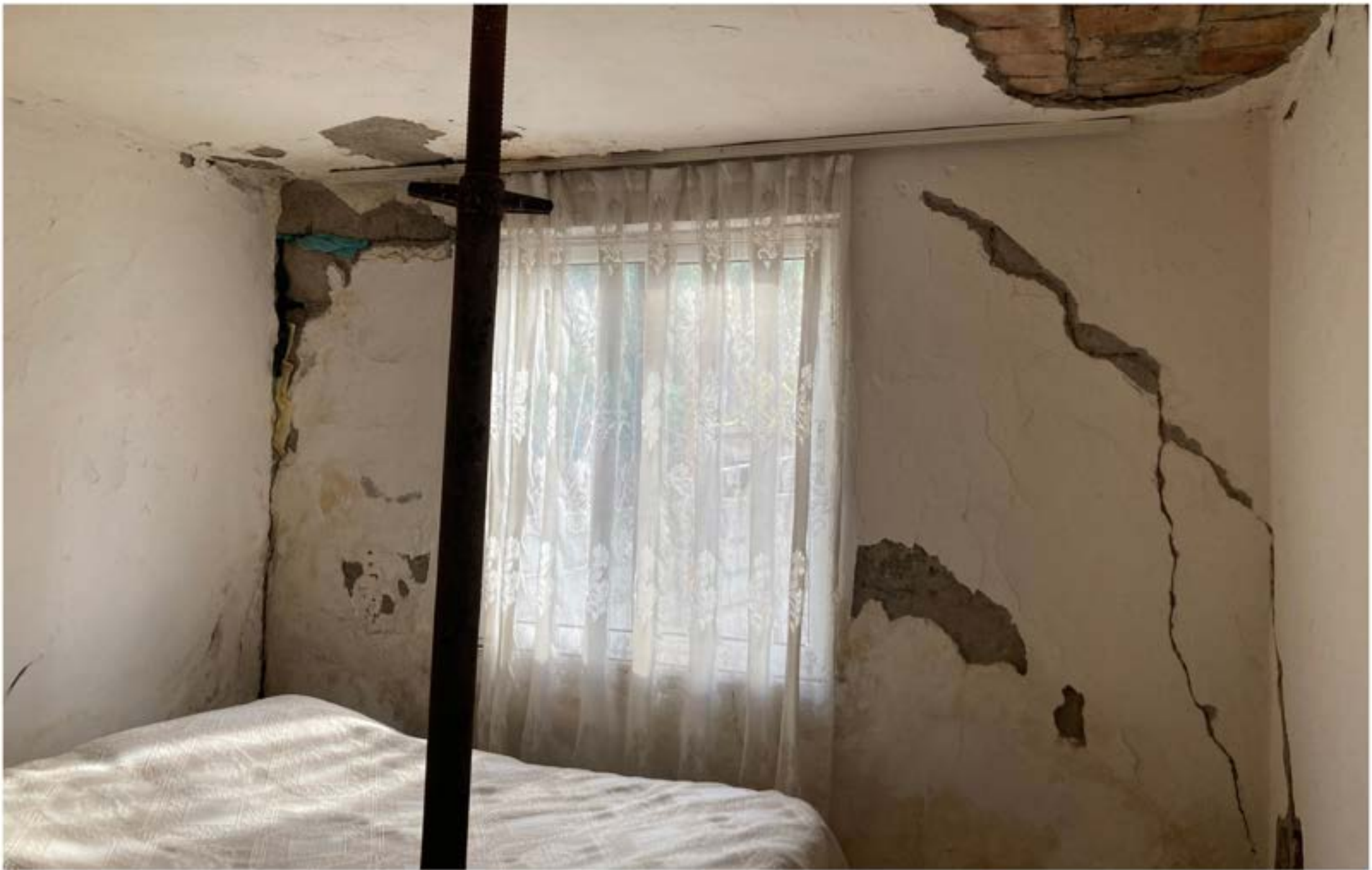
Figure 7 - A women's home in Zharrëz allegedly damaged by induced seismic activity (own photo).
