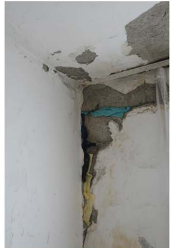
Figure 24 - Large crack in Fiqerete Gremi's bedroom wall, stuffed with rags and paper (own photo).
