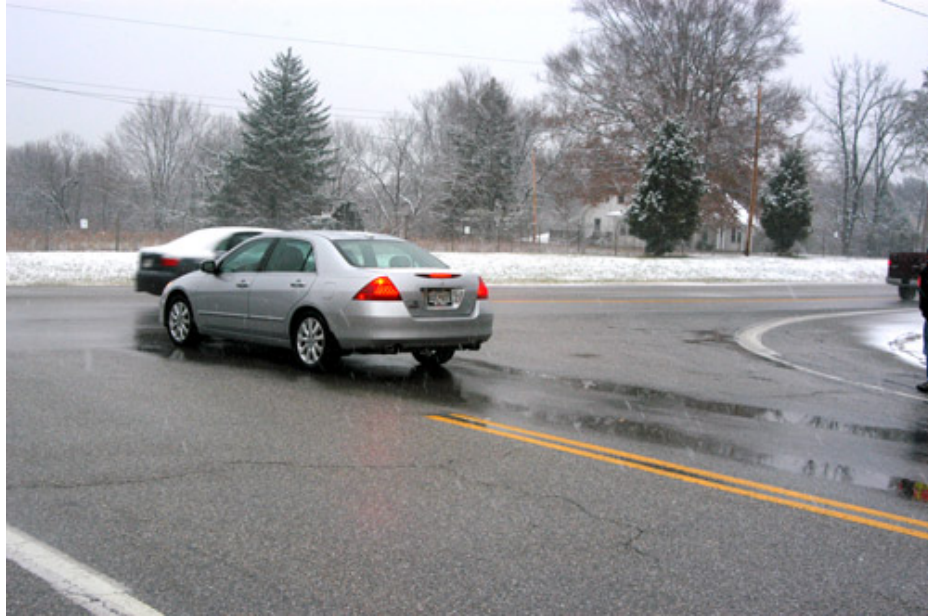
Figure 2: Water collecting in ruts
