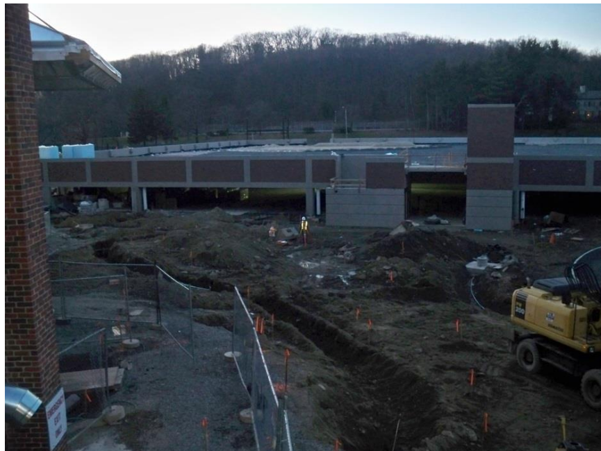
Figure 27 : View From Harrington, overlooking the construction Area, the Parking Garage is in the Distance
