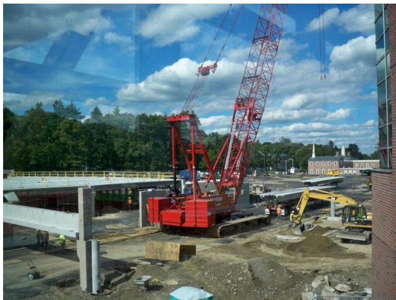
Figure 1: Looking out of the New Recreation Center to the construction of the parking garage and athletic fields (October, 2012)
