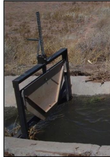
Figure 16: A check gate
