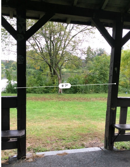
Figure C3: The gazebo closest to Salisbury Estates has a doorway that is currently 5' 7" in width. This doorway is the closest one to the lake and Goddard Hall gazebo.
