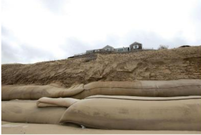
Figure 17: Exposed Geotubes in Sconset. (SBPF)
