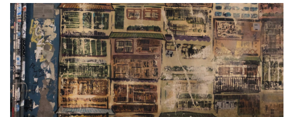
Figure 9. Old Townhouse Mural Deteriorating
