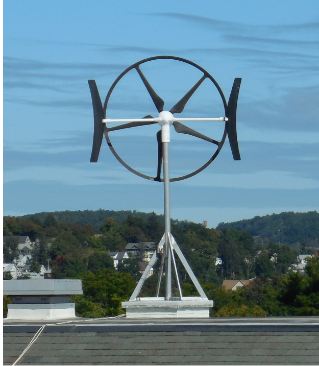
Figure 1: SWIFT Wind Turbine on Roof of AK
