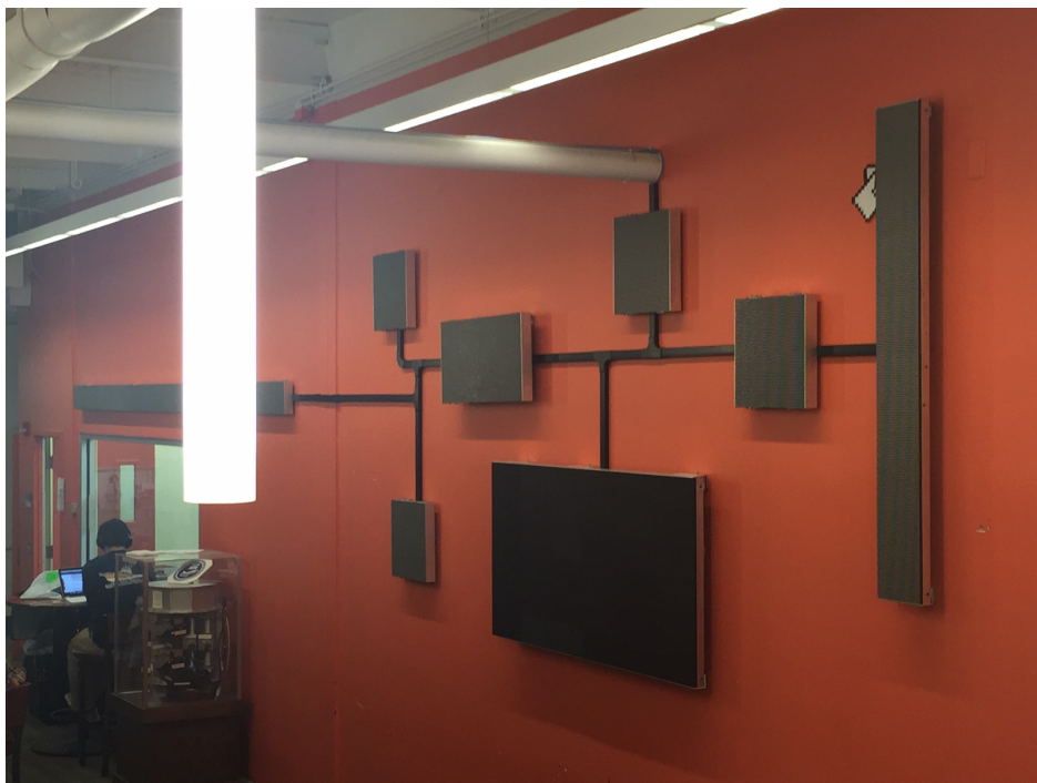
Figure 80: Power Panel in Pumpkin Lounge
