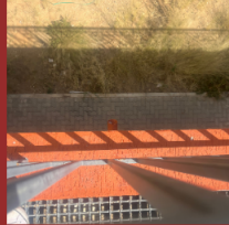
Rainwater Discharge Pipe
