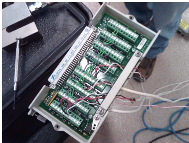
Figure 15: Wiring of strain gauge to signaling conditioner.
