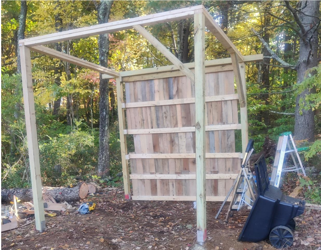
Figure 13: the Lodge with all the posts and top plates installed, as well as one of the walls and two of the braces
