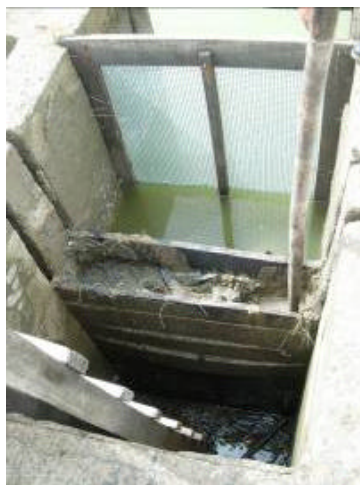
Figure 4-13 A water exit gate used for water exchange.
