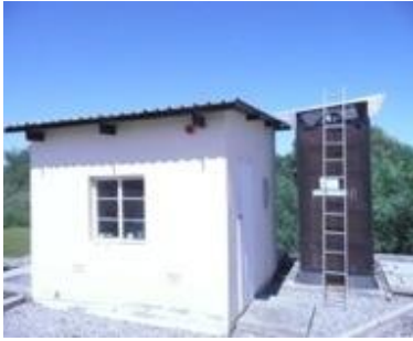
Figure 10: Main Station Trickle Filter & Septic System
