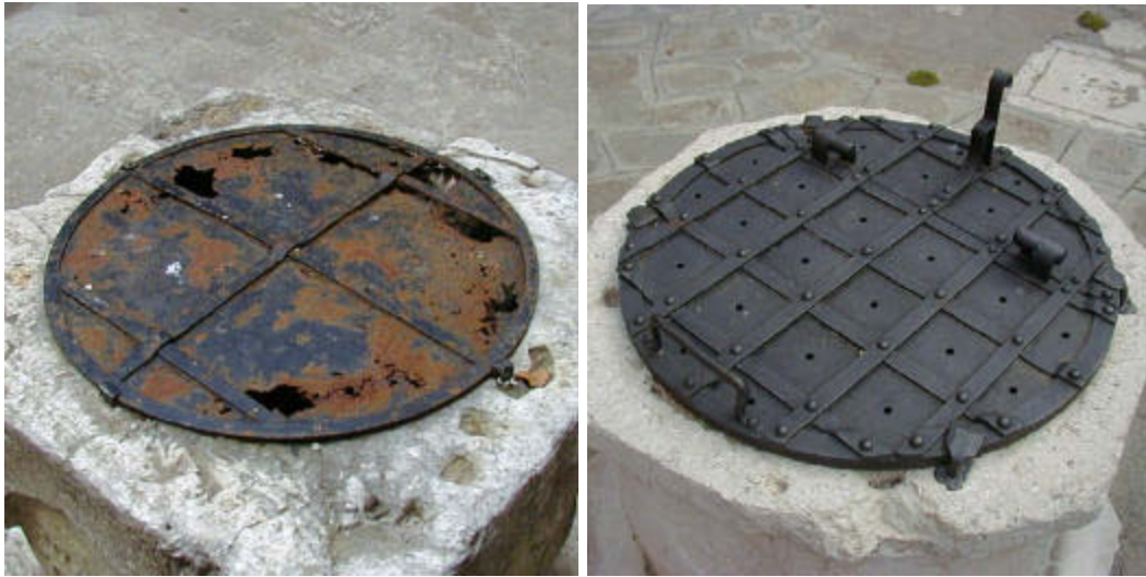
Figure 5-10 Lids in Bad and Good Condition
